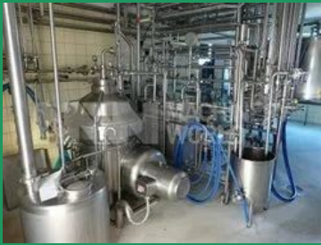
Milk Processing Plant And Machines
