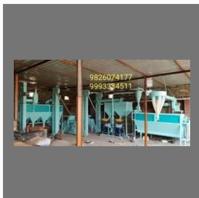
Flour Mill Plant
