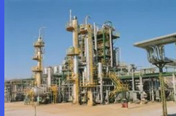
Industrial Distillation Column
