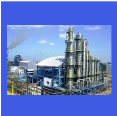
Industrial Distillation System
